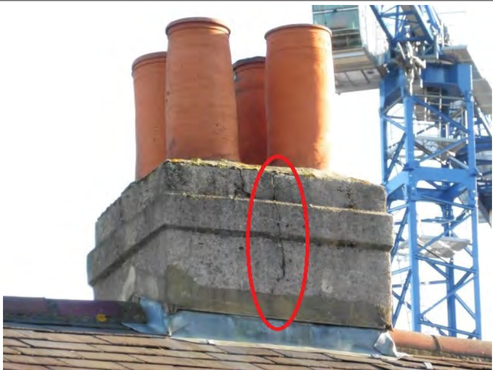
Central stack viewed from the front
