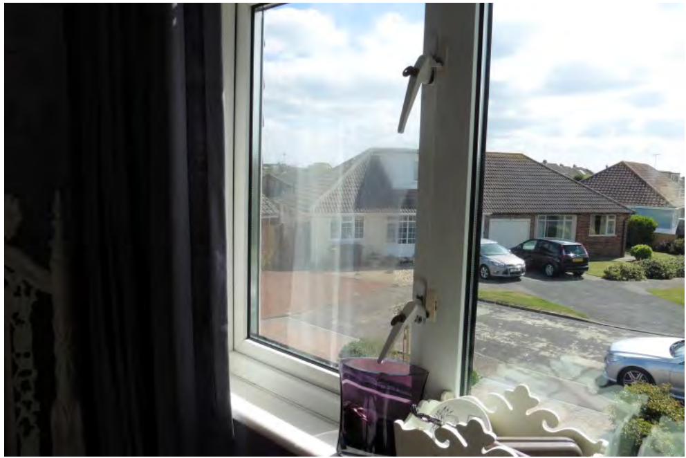
Bedroom 1 casement window panel blown
