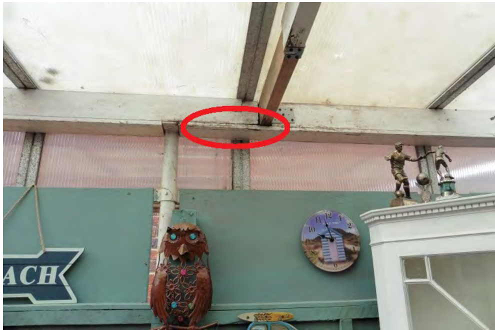
Possibly rotten timbers in the lean-to
