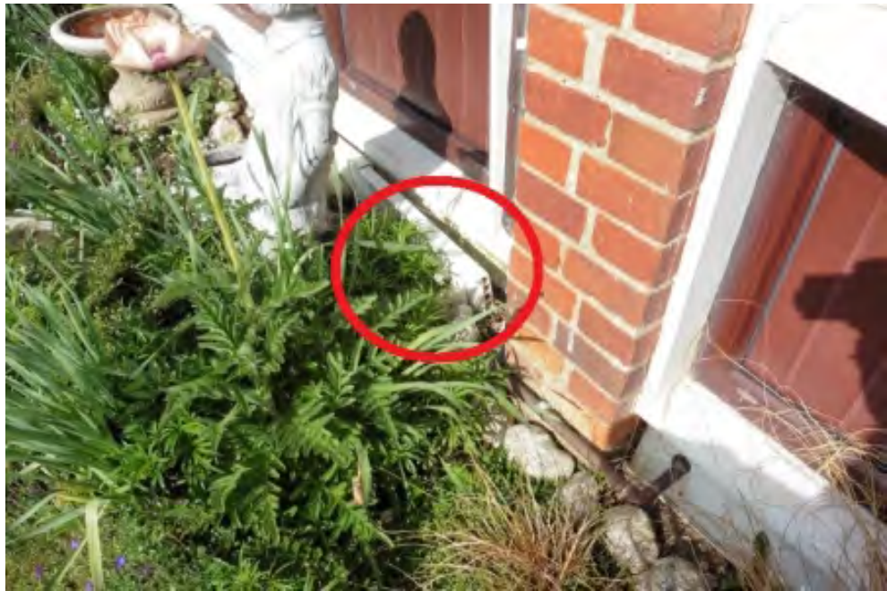
Loose plastic trim at the front
