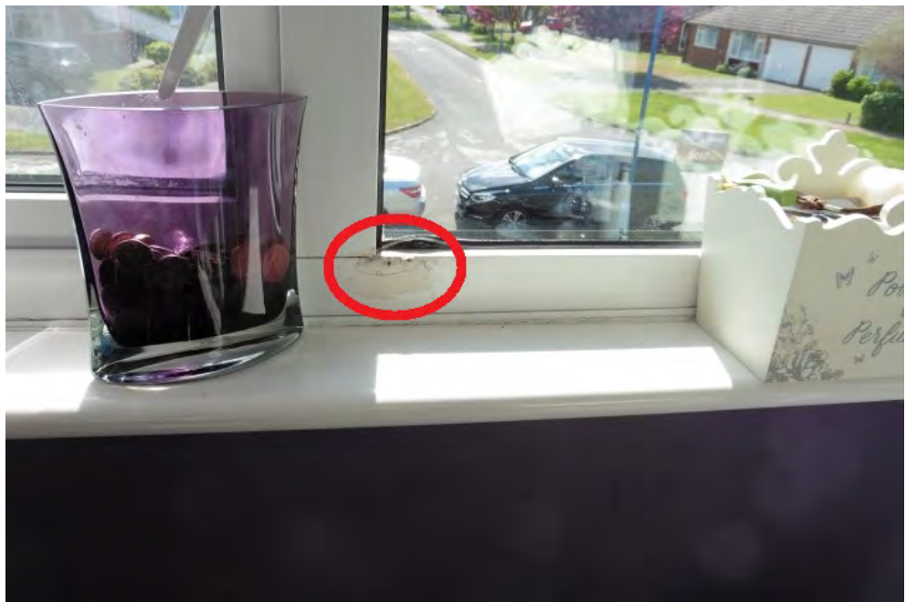
Damage to frame and seal in bedroom 1
