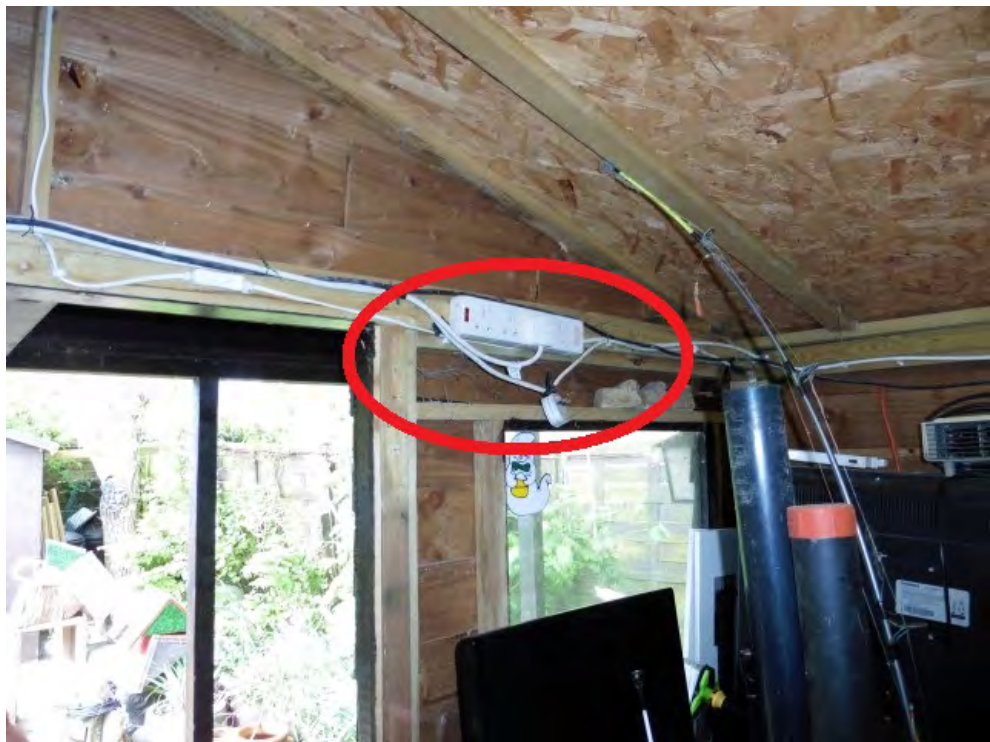
Poorly managed wiring in shed 4
